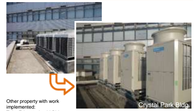
Renewal work of air-conditioning system: Enhancement of CS and reduction of environmental burden
