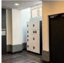
New parcel delivery lockers installed
